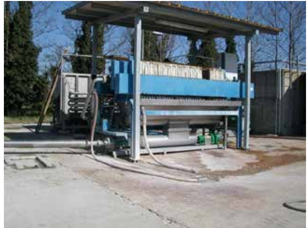
DHS pump Used after filter press for the recycling of the dried sludge.
