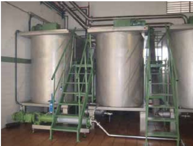
DN pump Used for transferring of pulp/olive paste.
