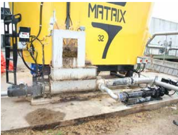
DHS-T and DN pump Transferring biomass to the digester with phase liquid injection.
